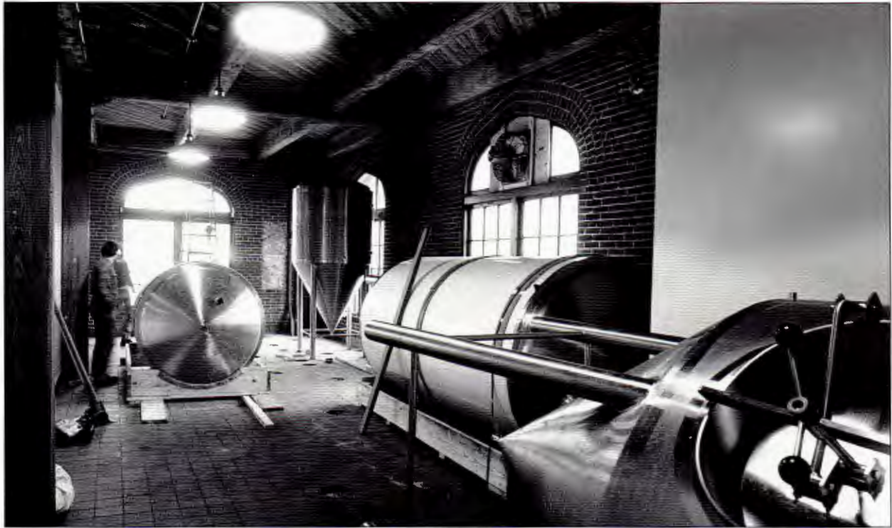
Installation of equipment at The Saint Louis Brewery, the city's first micro-brewery. Photo by Suzy Gorman.
