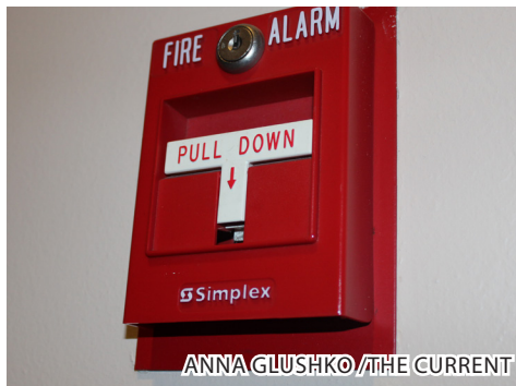
Fire Alarm on 2nd floor of MSC
