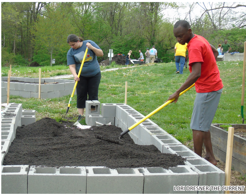
While some students level off the planters, others heft the soil into and out of the wheelbarrels
